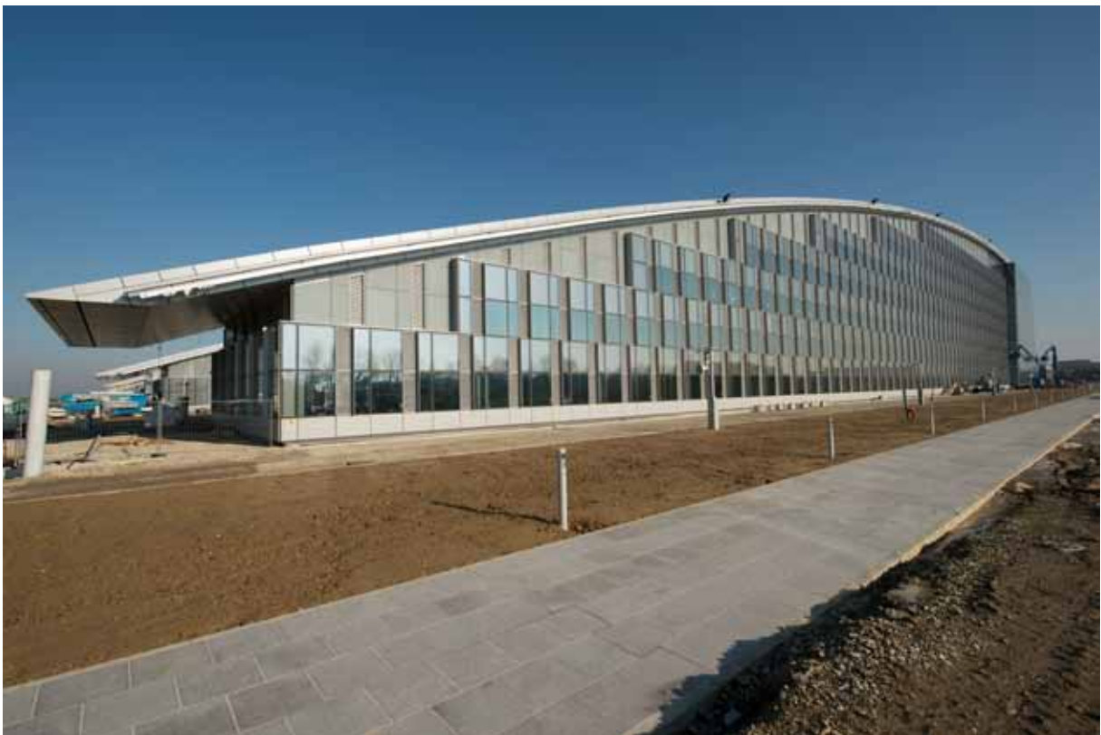
The new seat of the NATO headquarters in Brussels (Evere) under construction.
